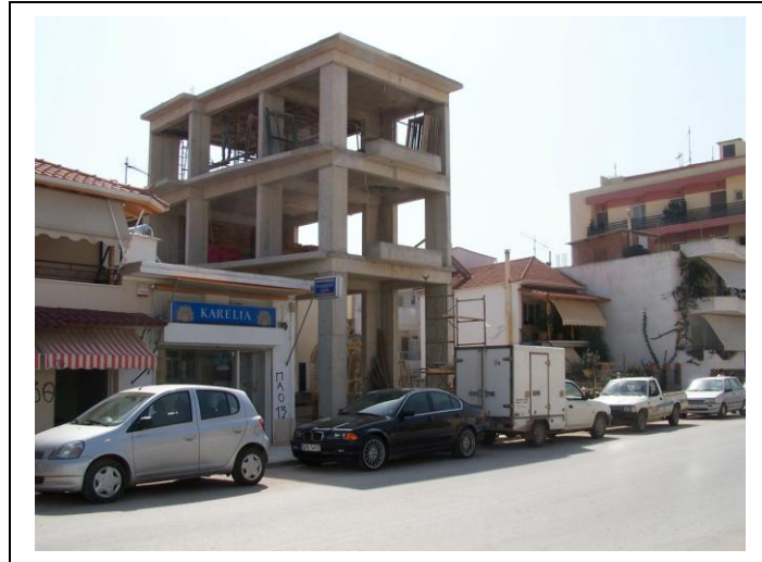
Fig. 3. A new block of flats (2003-2004) on Irinis Avenue eliminates the small public garden-plot.
